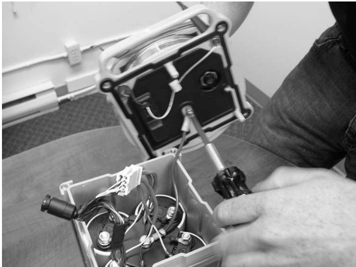
Figure 11-11: Re-attaching the Ground Strap
